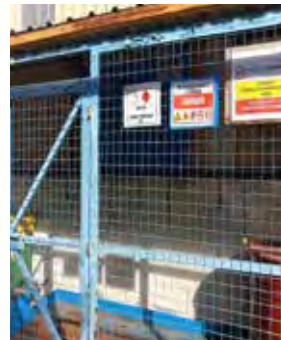
Spent Hydraulic Oil Storage
